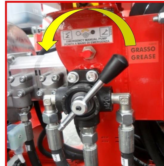
Picture 21: manual pump tap to be turned to the left.
