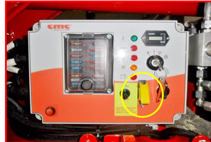
Picture 52: emergency bypass lever.
