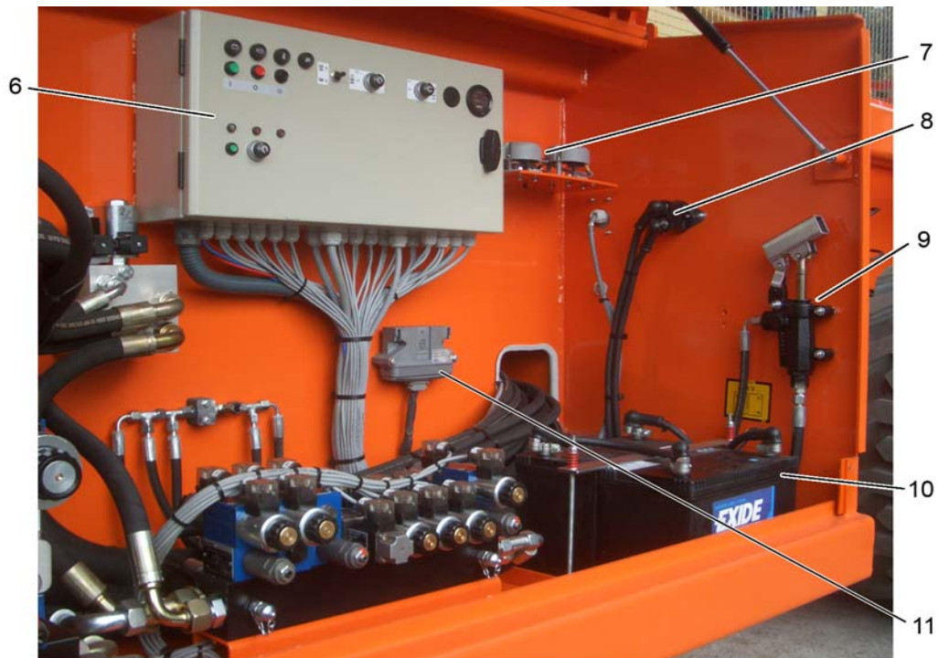
Valves and generator
